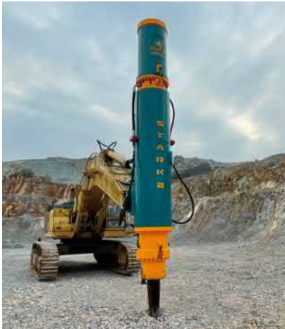
HHR100 Commissioning at jobsite
